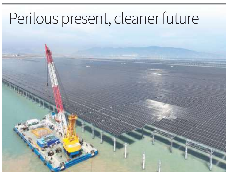
Towards sustainability: Solar panels being placed at the CNNC Tianwan tidal flat photovoltaic power plant in Lianyungang, in China's eastern Jiangsu province, on April 19.
