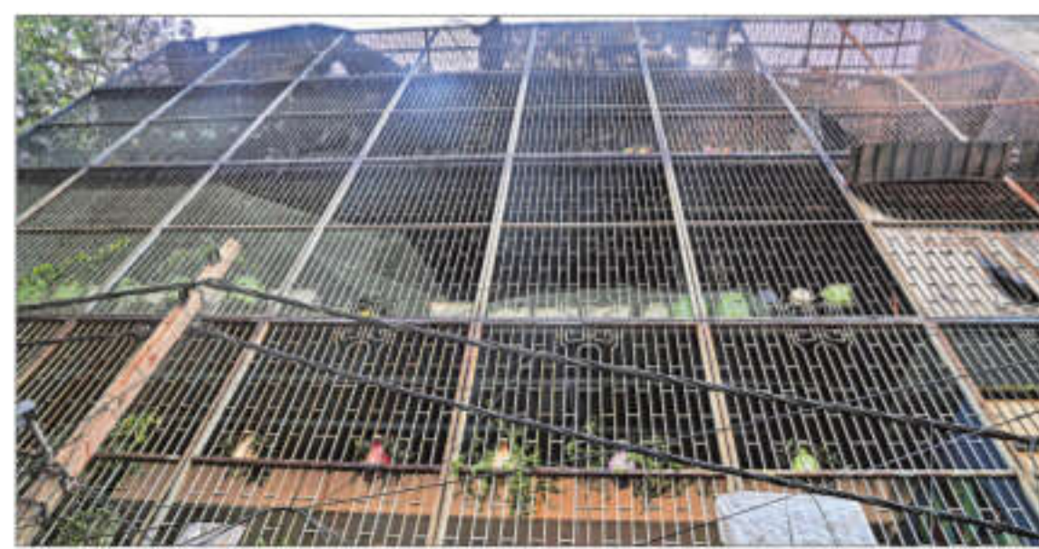
REAR ENCASED IN GRILLS: The flats at the back have enlarged their living spaces with cage-like extensions. The fire broke out at the back of the building. The strong, tightly packed grills prevented both escape and rescue.
