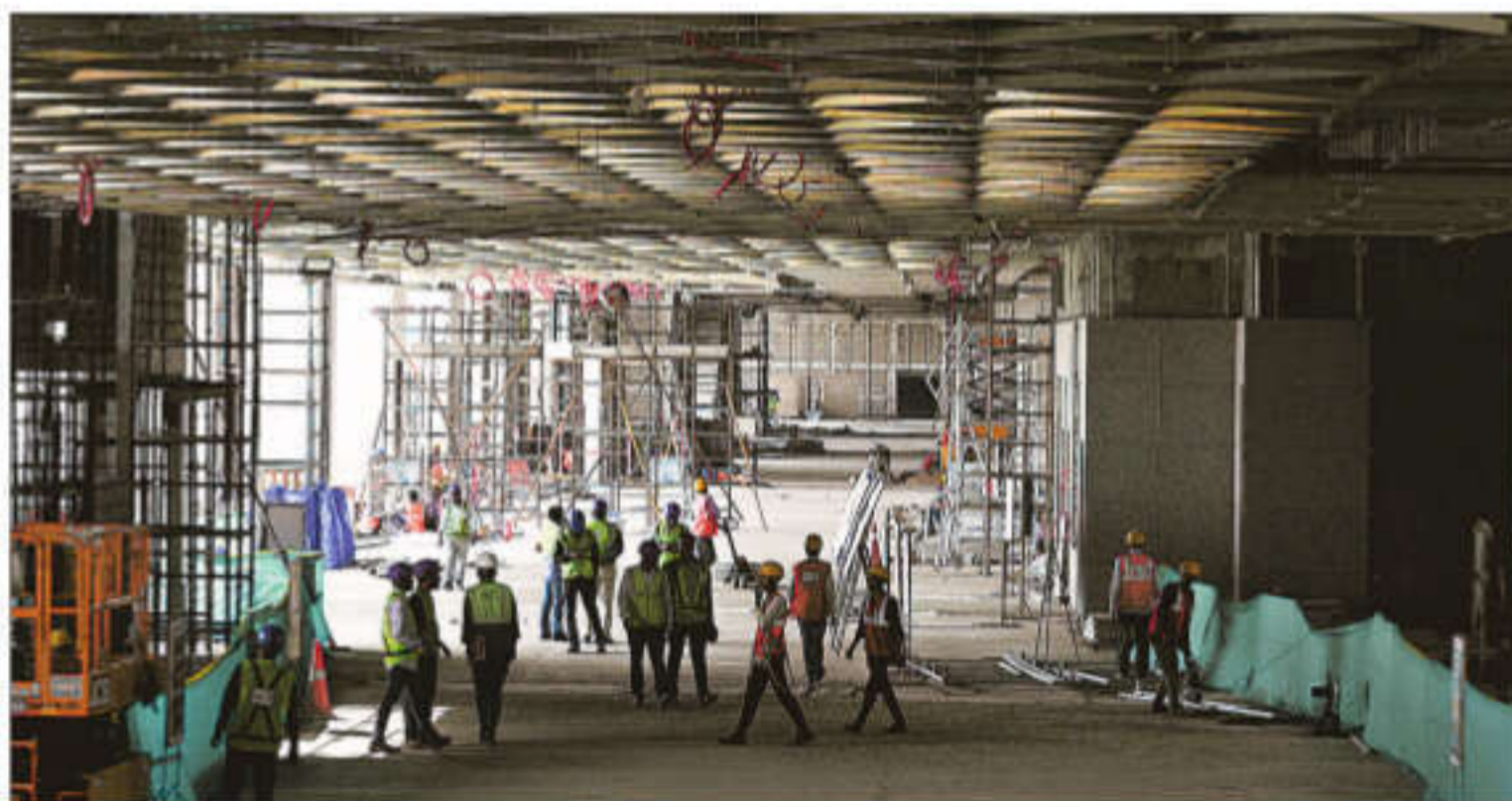
(Top) At Vikhroli in Mumbai, one of the many tunnels through which the Mumbai-Ahmedabad high-speed line will pass; work on at the Ahmedabad station of the bullet train
