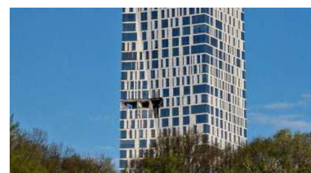
High-rise tensions: The damaged facade of a high-rise building following a drone attack in Moscow on Monday. REUTERS
