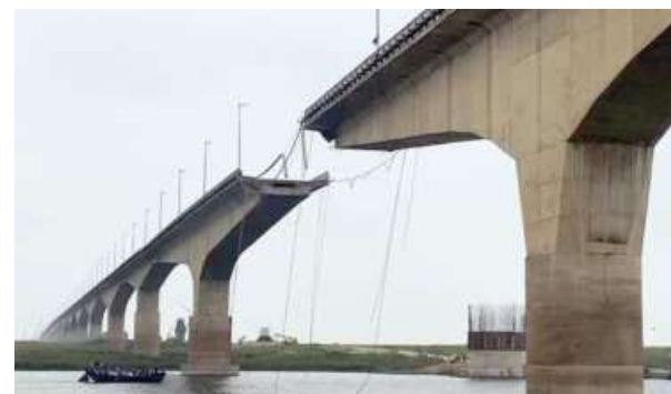
A slab of the Vikramshila Setu bridge collapsing into the Ganga river in Bhagalpur on Monday. ANI
