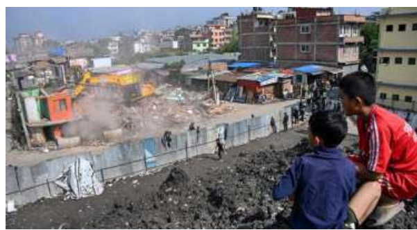
Nepal's newly elected Prime Minister Balendra Shah defended on Monday his push to clear informal settlements from stiff criticism by rights groups, in rare public comments since assuming office. Officials last month began demolishing squatter settlements home to thousands of people on government land in Kathmandu. AFP
