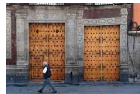
A person walks past two uneven doors showing a sinking building in Mexico City in July 2016. AP
