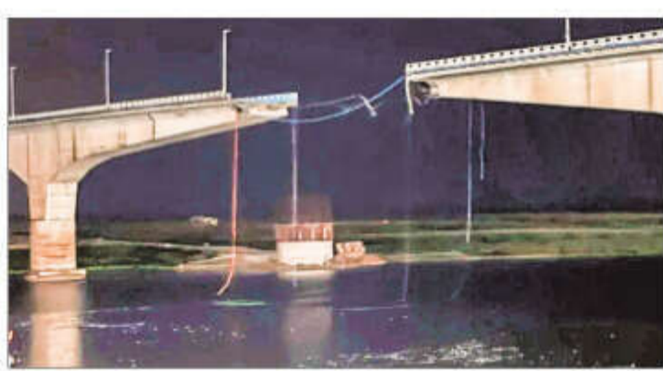
The partially damaged Vikramshila Setu in Bhagalpur on Monday. PTI
