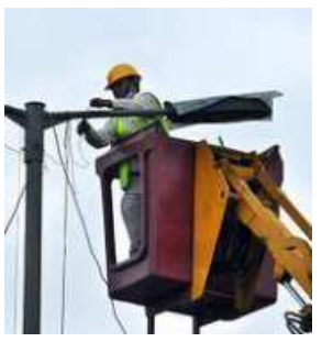
Nearly 96,000 street lights will be replaced before Deepavali, said the CMO. FILE PHOTO
