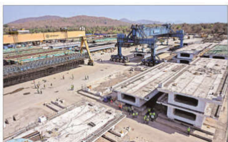
Sakhare village is one of the nine casting yards in Maharashtra, set up along the rail corridor to make girders. SANKHADEEP BANERJEE
