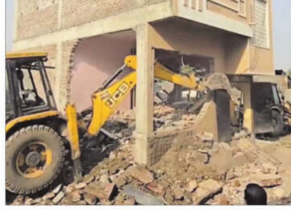
Hanif Khan's residence was demolished on May 13 by the Chhatrapati Sambhajnagar Municipal Corporation. FILE
