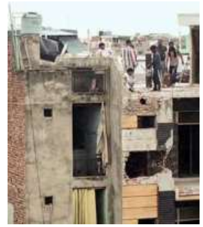
MCD officials carrying out demolition work in Uttam Nagar on Thursday. ANI
