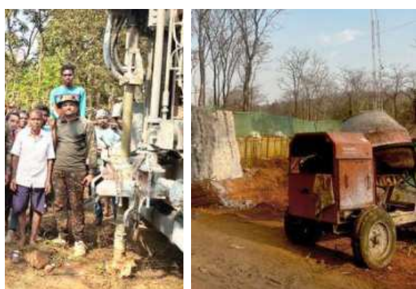
An electric borewell has been installed in Binagunda. More civic works are under way. SPECIAL ARRANGEMENT, VINAYA DESHPANDE PANDIT
